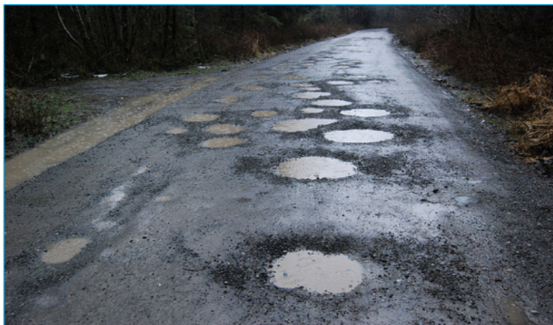
Fig. 16.10: A section of a road with potholes
