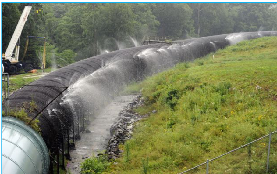
Fig. 16.11: A leaking pipe
