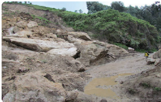
Fig 3.23 Land slide blocks at Mukamira Ngororero road
