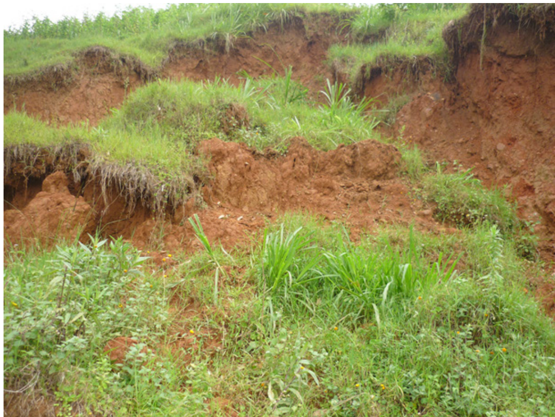
Figure 7. 128 Landslide in Gakenke district
