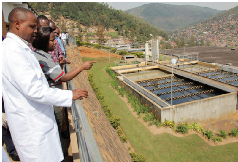
Yanze water treatment plant (Kigali)
